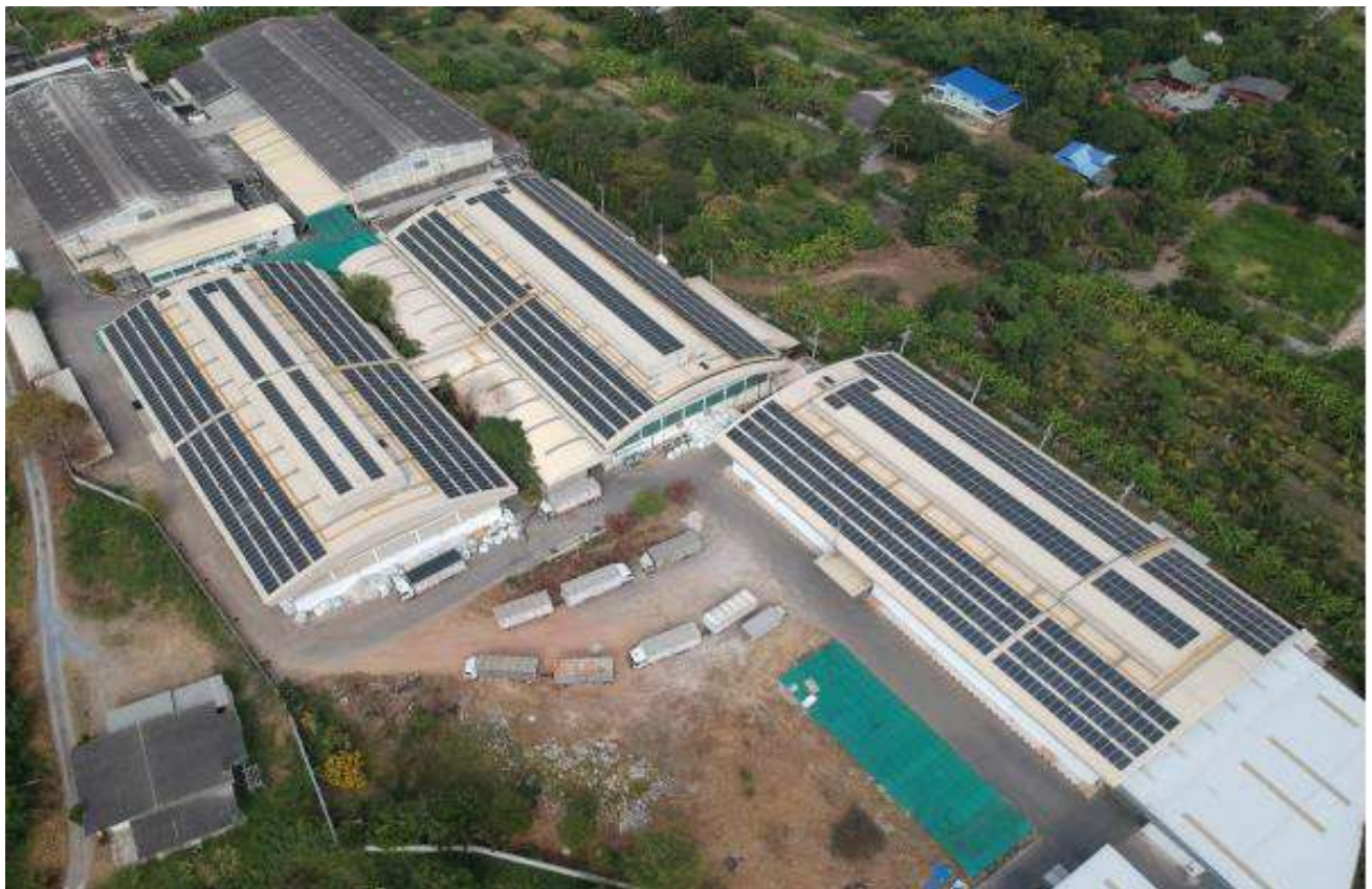
Installation of solar panels on the roof of the company's production building 3 buildings
